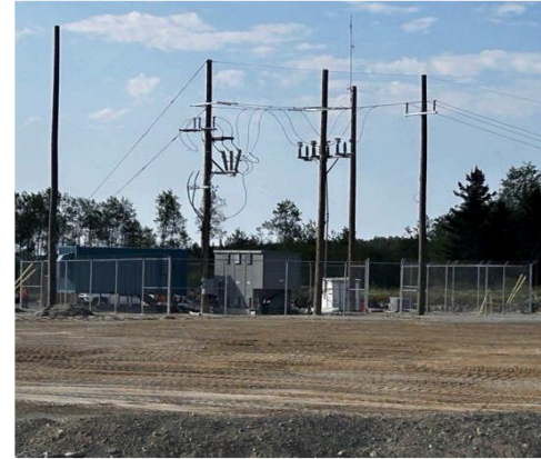
Hydro and Fiber Optic Line
